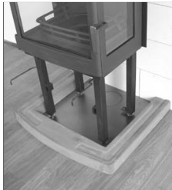
Fig 9 Put the base of the concrete casing in place – the marks in the metal plate indicate the right position (see Fig. 4). Check that the base is level and horizontal.
