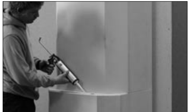
16. If you are going to fit tiles, move on the Photo 29. The foot-moulding and mantelpiece décor below (Photo 17) and above (Photo 18) the hearth are fixed in place with the silicon adhesive supplied. Use a spirit level to ensure they are horizontal.
