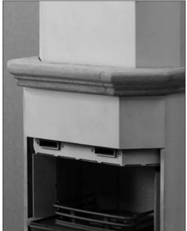
18. Fit the mantelpiece and fix it in place with silicon adhesive. Check that it is horizontal.
