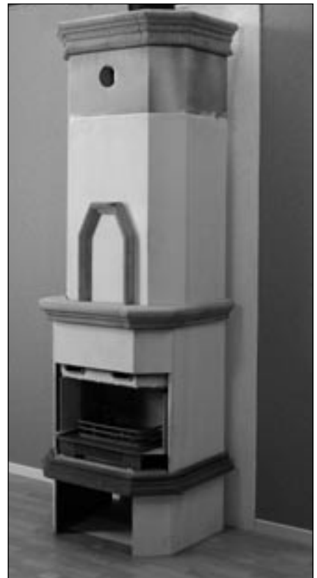
27. The tiled stove is ready for the application of an external finish.
