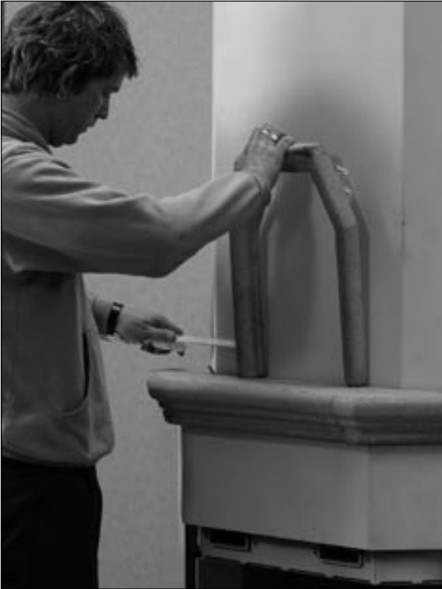
24. If you want to fit a niche, check that it is properly centred and attach it with silicon adhesive.
